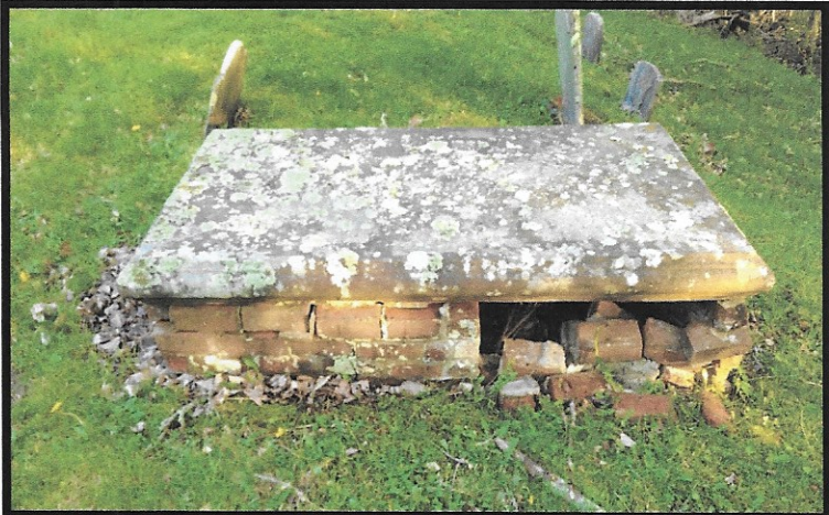
The crypt in state of disrepair
