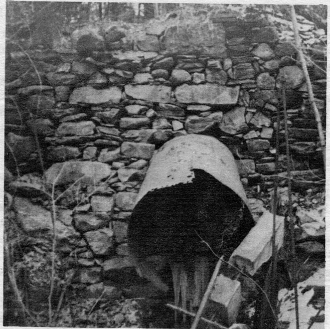
Houghton Grist Mill foundation and four foot pipe flume to water wheel
