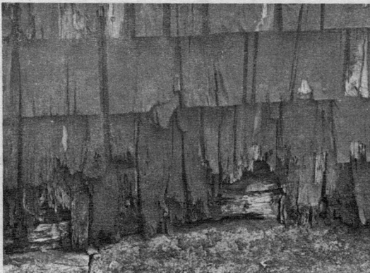
Typical exterior areas requiring restoration.
